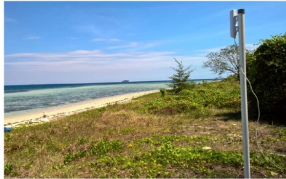
Fig. 2. Installation of Ubiquiti Device.
